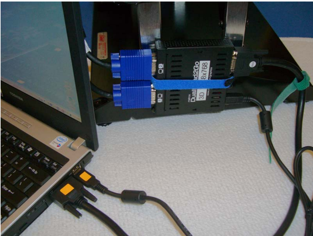
Matrox DualHead2Go strapped to the side of the Chief Stand and plugged into the laptop (cables marked in orange). Cables to the projector have the large blue connectors.
